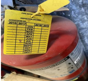
Location Shalimar (Kingston): Outdated fire extinguisher last serviced in July 2017
