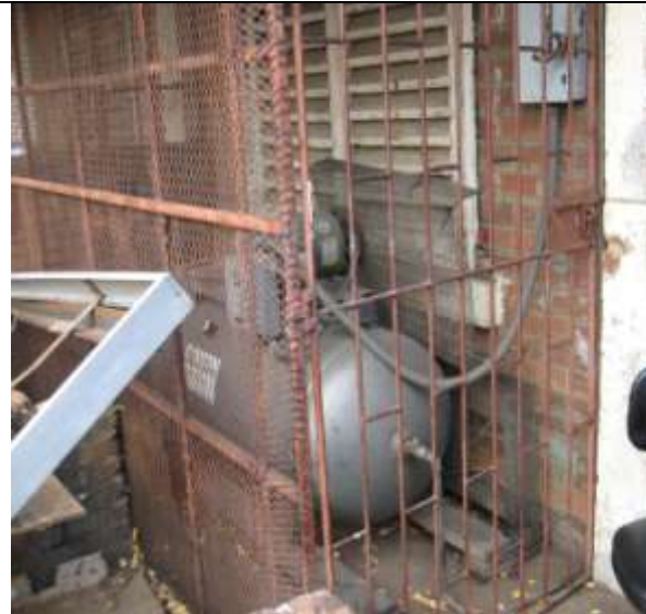
Compressor at Welding Shop – out of order
